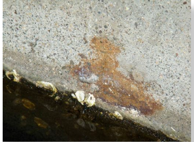
Evidence of corrosion on the concrete hull at slip B3.
